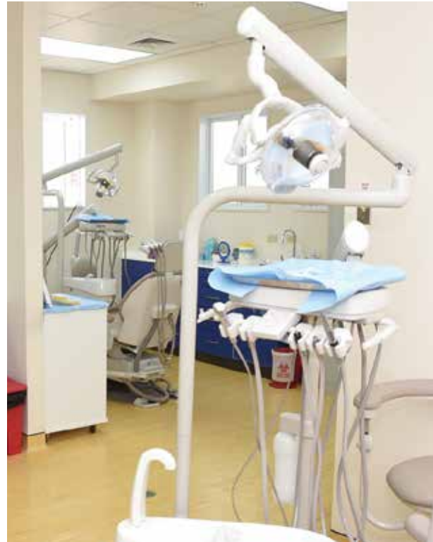
Upgraded facilities at the Arima Dental Clinic will provide students with practical opportunities and the public with low cost dental care.
