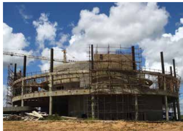
The Moot Court under construction in early 2014 at the The UWI St. Augustine South Campus, Penal-Debe.
